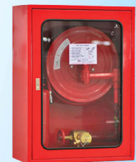
Fire Hose Cabinet ( Complete Set )
